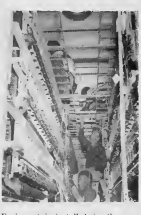
Equipment is installed in the new telephone exchange building.
